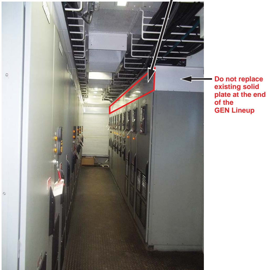
Figure 5: Power House Existing Cabinet Cover Plates (above Gen Lineup)
