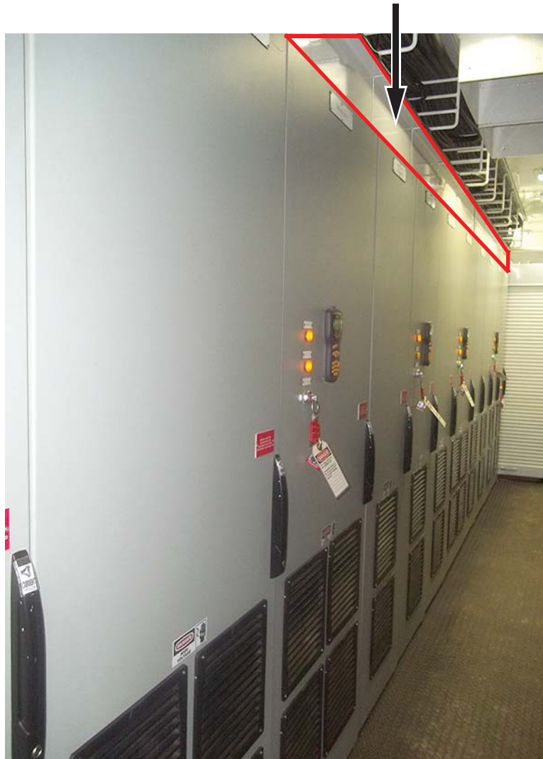
Figure 7: Power House Existing Cabinet Cover Plates (above VFD Lineup)
